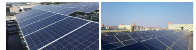
▲ Solar power facility at Changshin Vietnam ▲ Solar power facility at Changshin China
